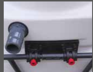
Waste water drain cock
